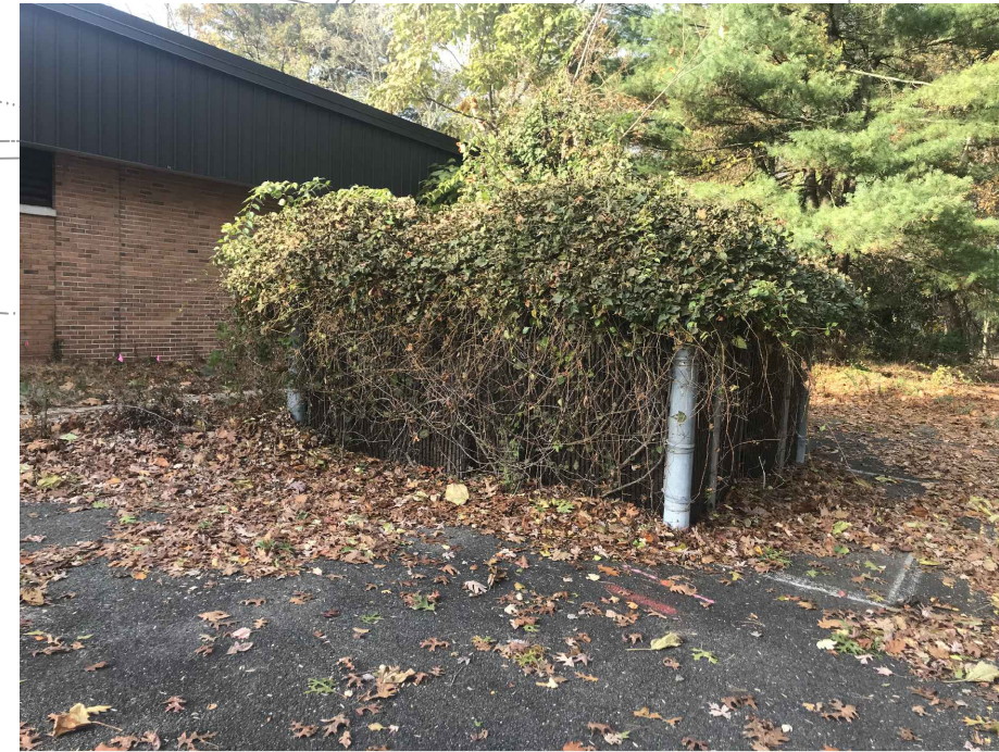
VIEW 4 - TRANSFORMER TO BE MAINTAINED
